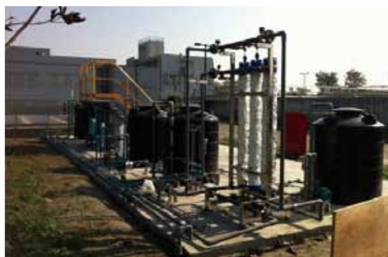
⊕ Erlin Sewage Treatment Plant: effluent water provides Erlin High School with Secondary domestic water.
